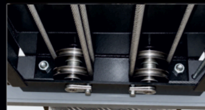
Under-runway cables and pulleys.
